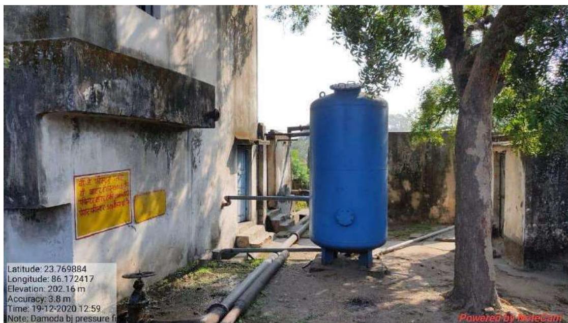
FILTER PLANT IN THE MINE AREA
